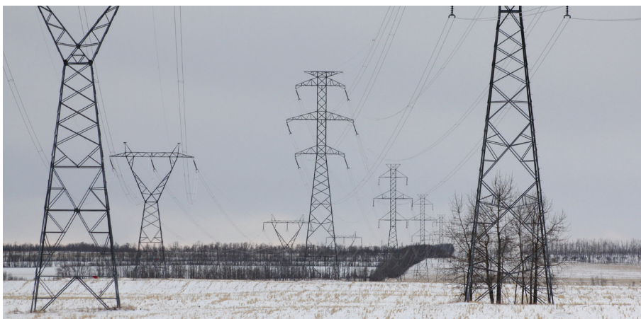
Pictured, transmission lines east of Innisfail.
