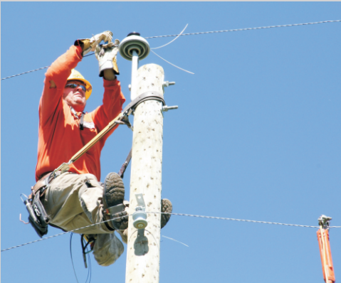
CAREA Power Line Technician Darcy Wood works to string up a new line after a tornado, which touched down near Innisfail on Thursday, July 7, snapped lines and a power pole.
